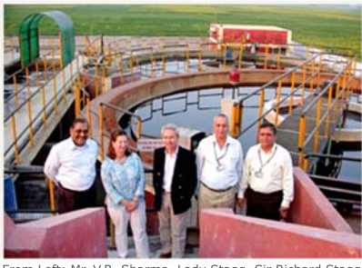
From Left: Mr. V.R. Sharma, Lady Stagg, Sir Richard Stagg, Mr. Rajesh Kapoor & Mr. Makarand Mehendale at the Obeetee Effluent Treatment Plant
